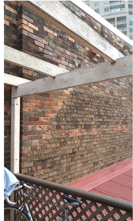
Figure 157: View of brick repairs to external wall of SBW Stables Theatre. Roof over kitchen visible.
